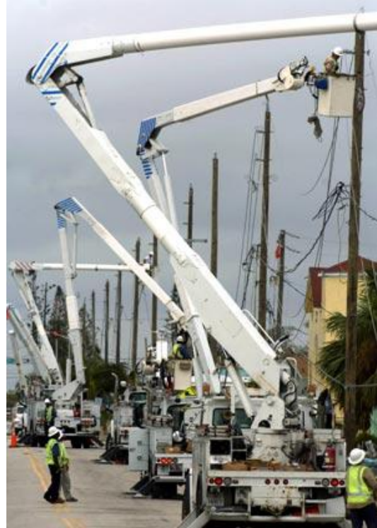
A crew of Dominion Virginia Power linemen from Virginia Beach, VA, operate a half-dozen bucket trucks on Martin Luther King Jr. Blvd in Boynton. (Staff Photo/Mark Randall)
